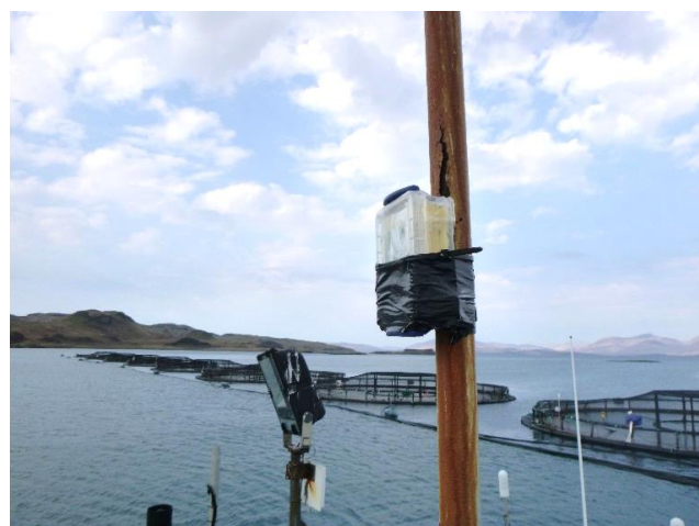
Figure 1B. Example of an AudioMoth in its box installed on a fish farm barge in 2019. © Texa Sim/SAMS-UHI.
